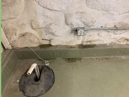
Basement water sensor
